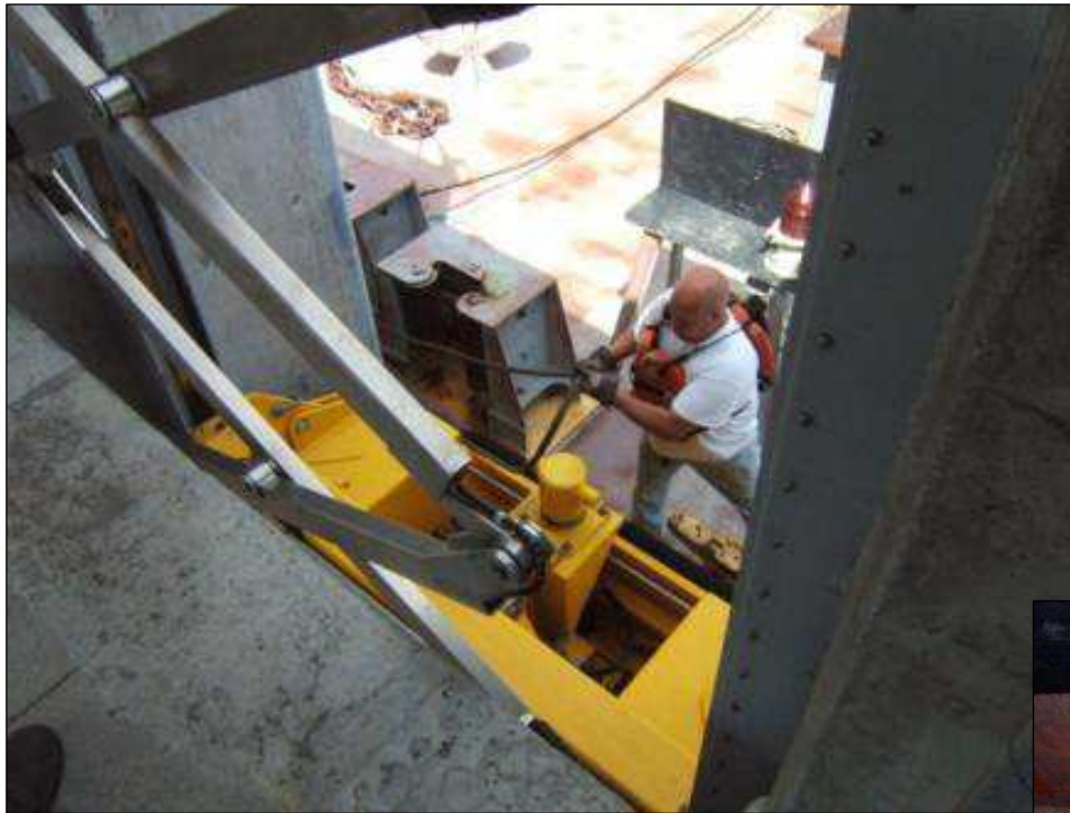
Barge of 1,500 tonnes securing to mooring bollard on top of the MoorMaster®
