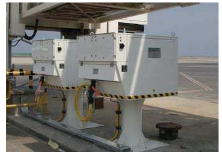
Specialised cable coils at Nice Airport.
