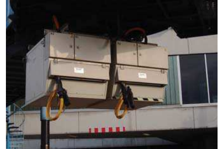
Dual coils mounted under a passenger bridge.
