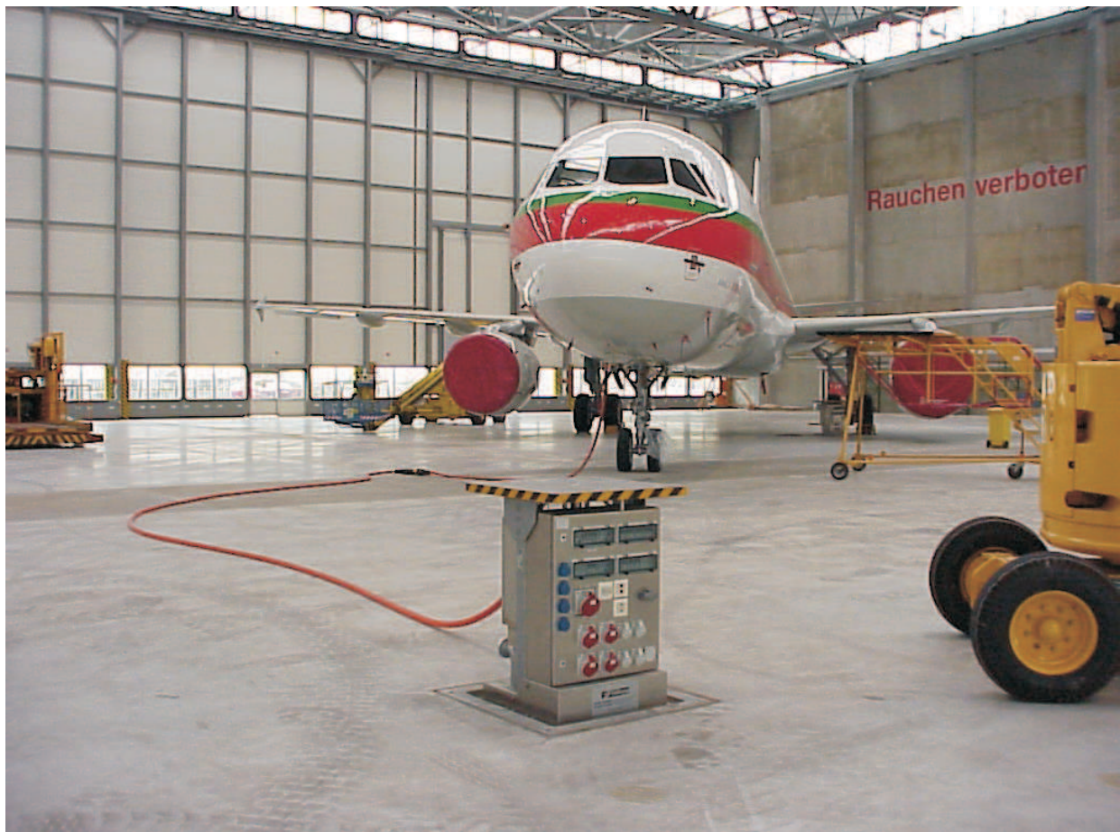
Fladung Hangar Pit at DASA (Airbus) in Hamburg
